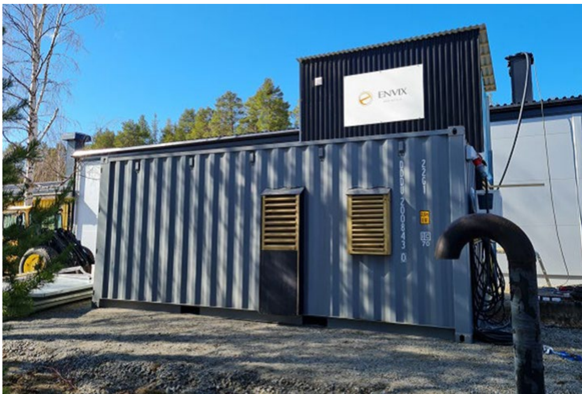
Figure 3. Photo of the E-peroxone pilot system at Lycksele sewage treatment plant.
